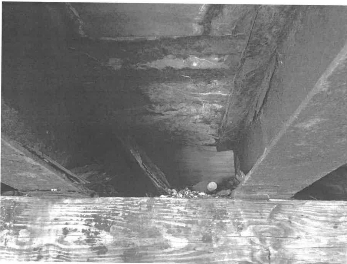
IMG_2122 Showing deterioration of concrete deck and steel beams.
