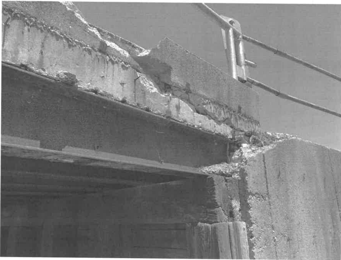
This picture shows the south beam at the time of the curb inspection.
