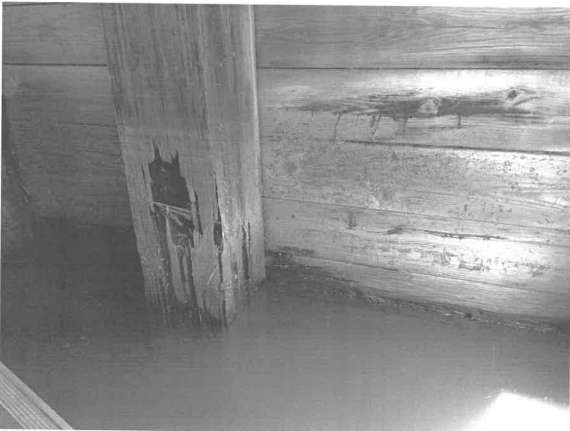
IMG_2108 Showing deterioration of timber pile.
